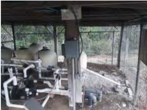
Pumps - 1 pump is by Pentair 3HP
